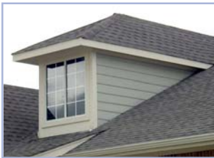
The deep overhang and lack of detail at the base of this dormer makes it inappropriate.
