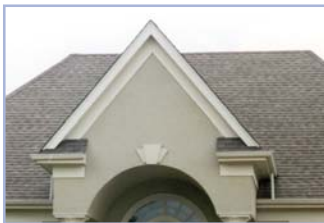
This steep gable with inappropriate rake details and oversized cornice returns is inappropriate.
