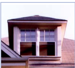
This hipped roof dormer is appropriately detailed with tight head, jamb and sill details.
